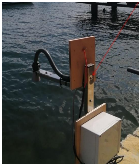
Figure 4: Station Alex3 (ATG)
