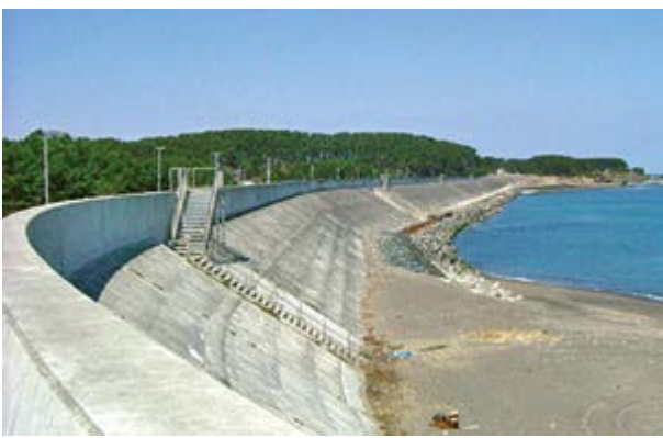
Sea wall with stairway evacuation route used to protect a coastal town against tsunami inundation in Japan. Photo courtesy of River Bureau, Ministry of Land, Infrastructure and Transport, Japan.
