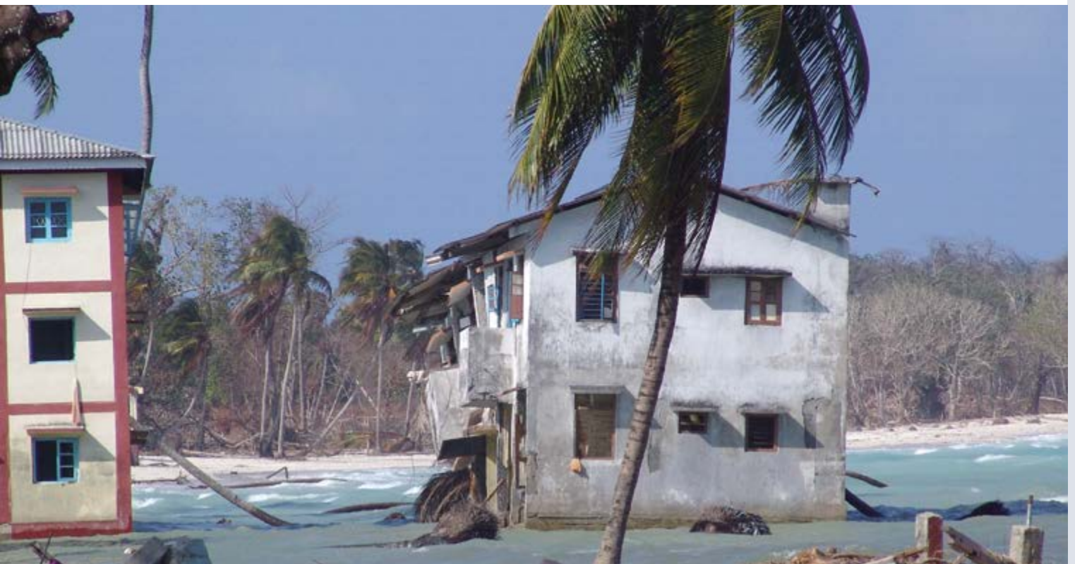
The 26 December 2004 earthquake resulted in 1.2 m of land subsidence in the Car Nicobar, Nicobar Islands, India, leaving houses that were once above sea level now permanently submerged. Photo courtesy of ICMAM, Chennai, DOD, India.
