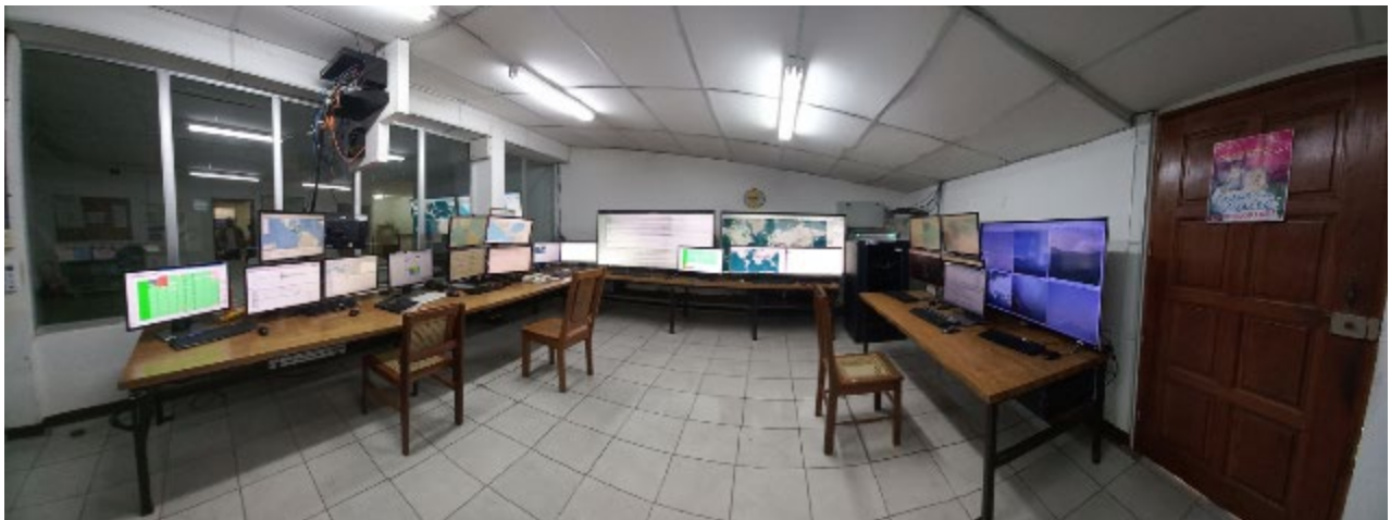
Photo 2. CATAC, Processing and Alerting Room
