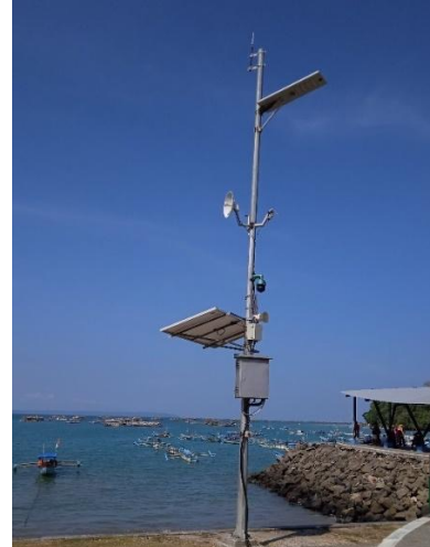
Smart Poles at four locations
