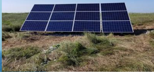
HF Radar solar power array in Texas.
