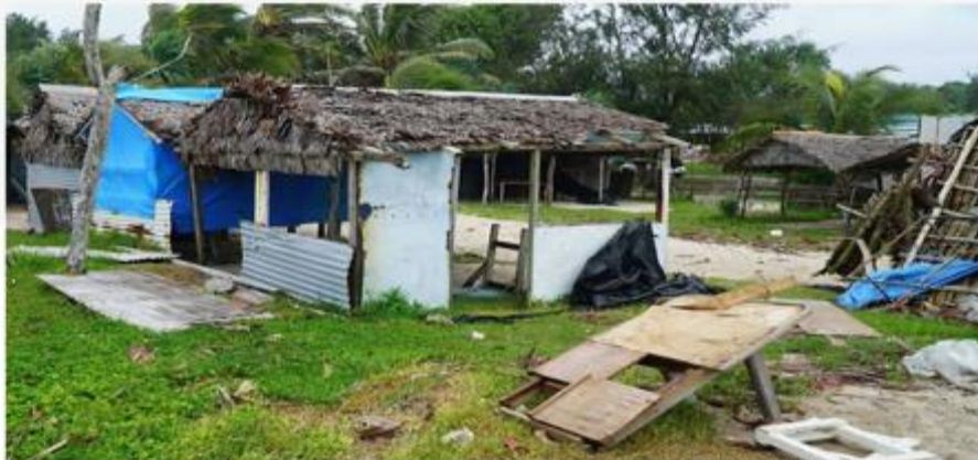
Badly damaged buildings are pictured near Vanuatu's capital of Port Vila after Tropical Cyclone Harold swept past Source: Getty Images
