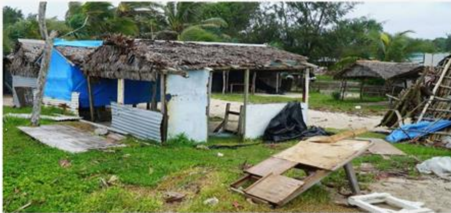
Badly damaged buildings are pictured near Vanuatu's capital of Port Vila after Tropical Cyclone Harold swept past Source: Getty Images
