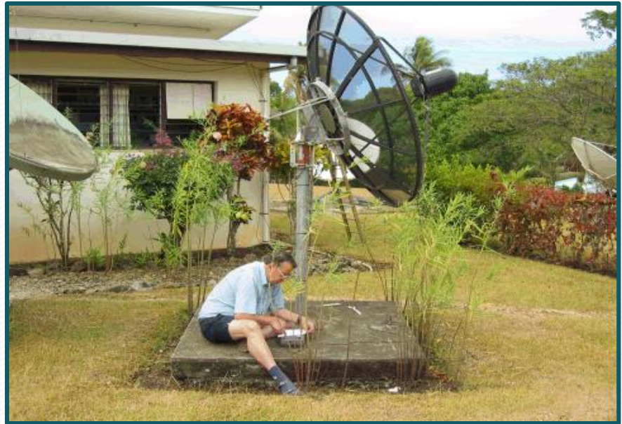
EMWIN C-Band Dish Antenna at Met Office, Port Vila, Vanuatu
