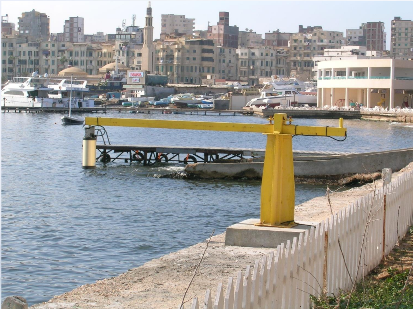
Radar gauge at Alexandria, Egypt installed with assistance from NOC, UK and IOC
