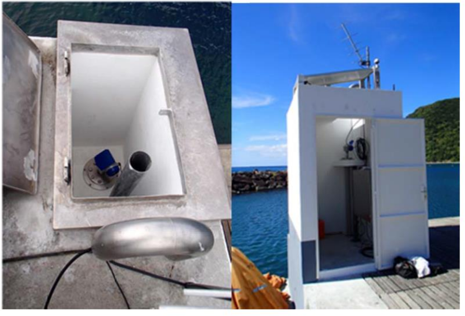
Time domain reflectometry radar gauge at Deshaies, Guadeloupe (stainless steel cable in a stilling well)
