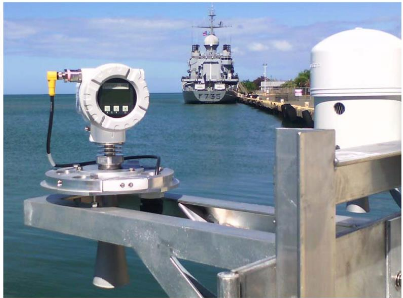
Two horn radar gauges (Waterlog H-3611) at Mayaguez, PR
